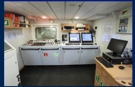
Engine Control Room Console for Anchor Handling Tug Supply Vessel
