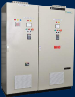
VFD Panel (355kw) for Philips Carbon Black
