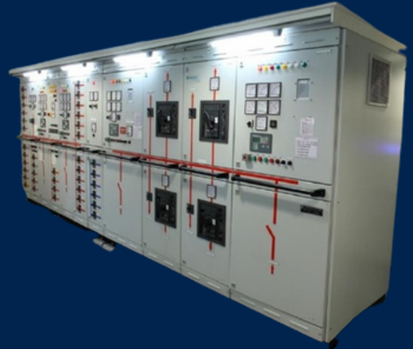
MSB (4000 A, 50kA) Certified by ABS for the biggest barge built by Cochin Shipyard for NPCC, Abu Dhabi.
