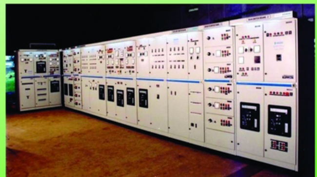
MSB for 1700 Cu.M Capacity Trailing Suction Hopper Dredger Certified by IRS for DCI
