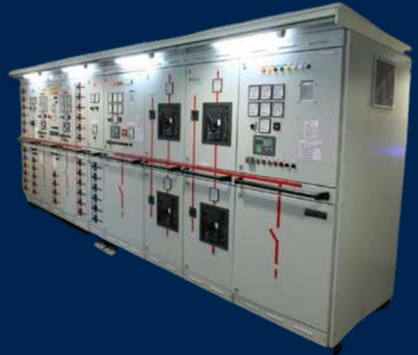
MSB (4000 A, 50kA) for the biggest barge for NPCC, Abu Dhabi.
