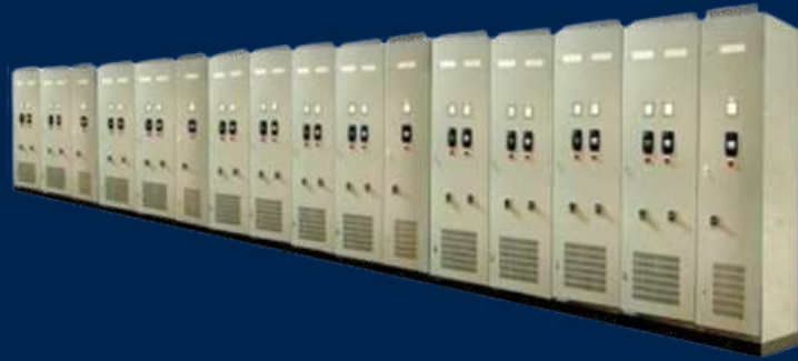
Auxiliary & Standalone VFD Panels (2.2kw to 200kw) for ITC , Kovai
