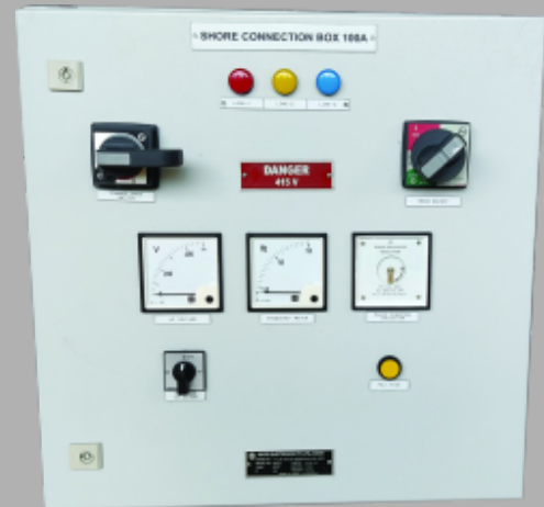
100A SCB for Inspection Barge Indian Navy Certified by IRS
