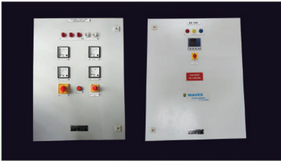
AC Switch Board for CIAL Vembanad Solar Powered Certified by IRS for Cochin International Airport Limited
