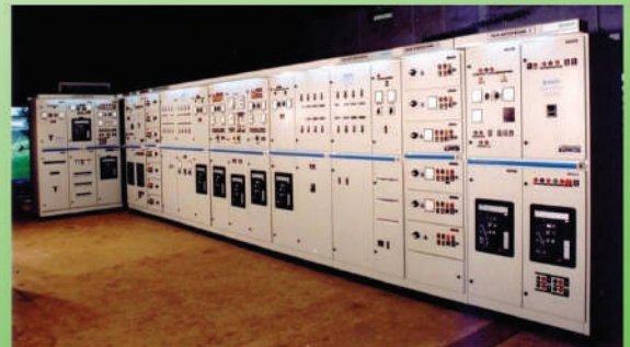
MSB for 1700 Cu.M Capacity Trailing Suction Hopper Dredger Certified by IRS for DCI
