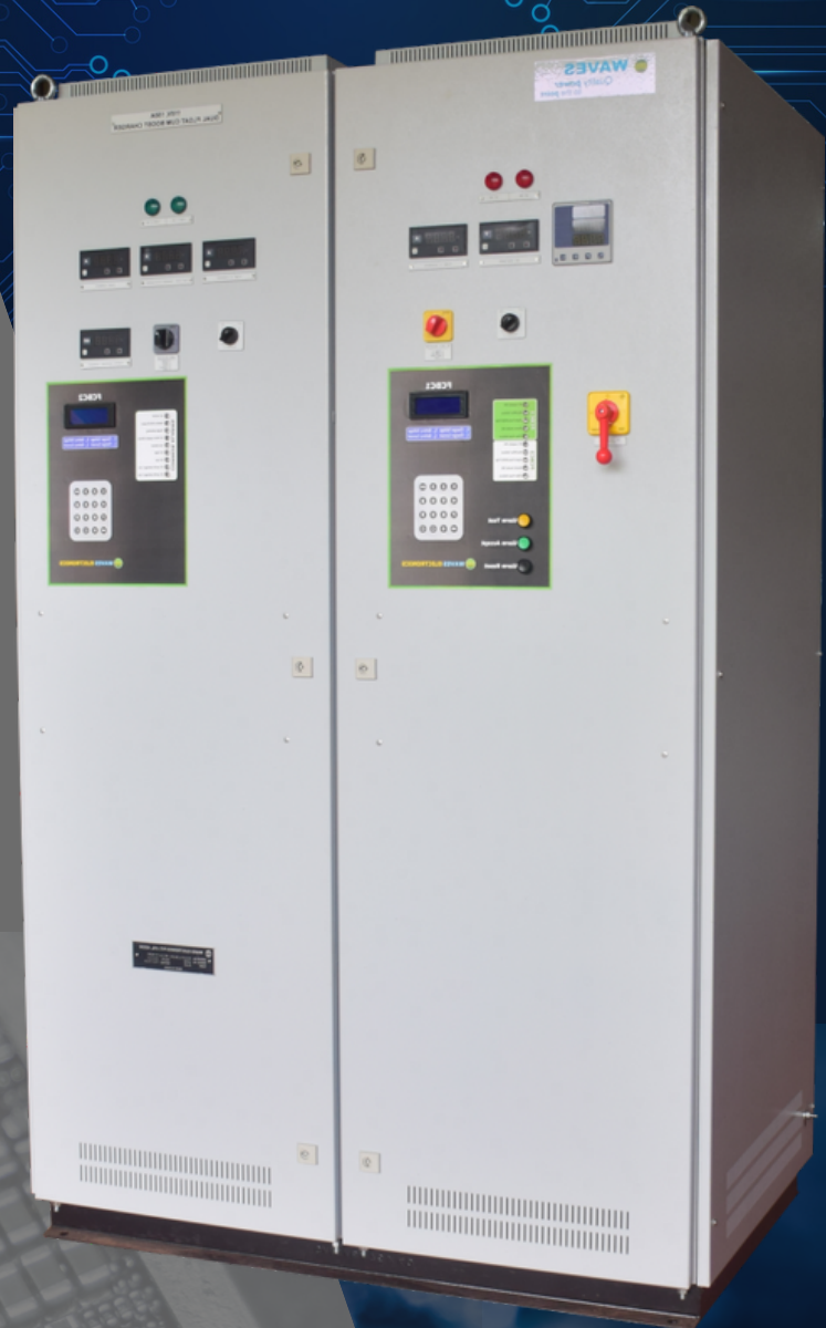
110V 150A Dual battery charger for Generating Station
