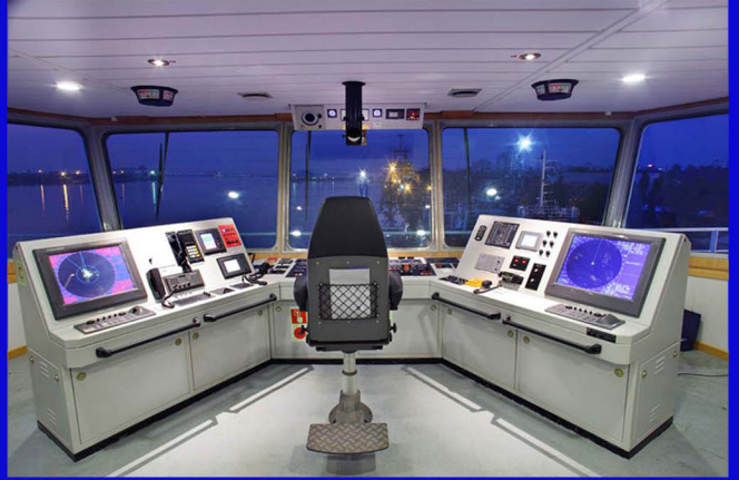
WHEEL HOUSE AFT CONSOLE OR 120T BP ANCHOR HANDLING TUG SUPPLY VESSEL ( SCI PAWAN )
