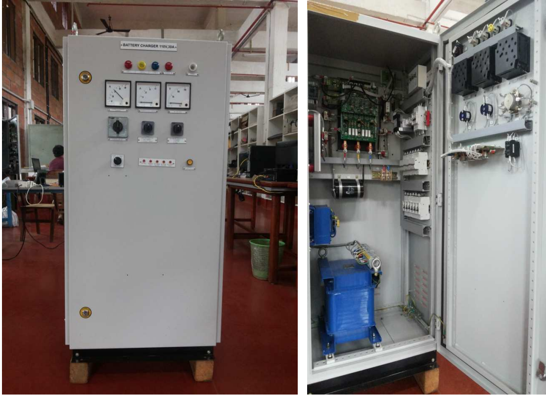
Figure 1: Three Pulse thyristor battery charger with remote Monitoring
